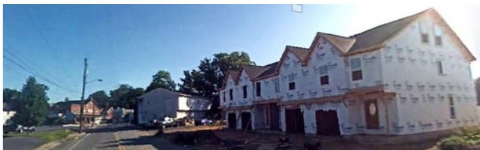
Townhouses under construction where Dewey's townhouse building burned to the ground. The parking lot for Cosmo's Restaurant is across the street. (Google Streetview, 2009)
